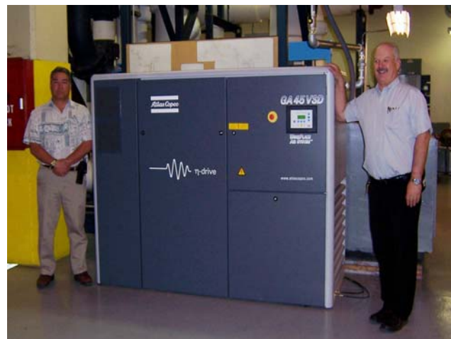
Don Apodaca and Steve Keltner with the New Atlas Copco VFD 60-hp Air Compressor
