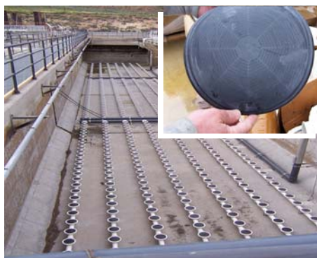
Fine Bubble Disk Diffusers in Aeration Tank
