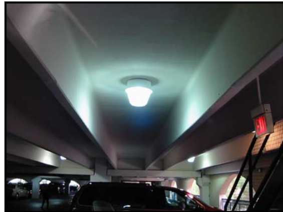
New CFL fixture
