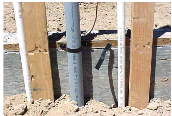
Figure 4 Conduit Support Strap Attached To Sill Plate
