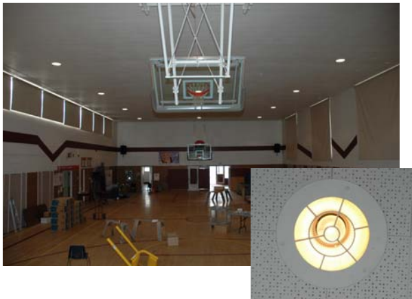
500 W Incandescent Fixtures in Gym
