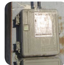
Photo of water damage.
