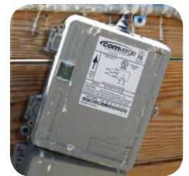
Photo of poor mounting.
