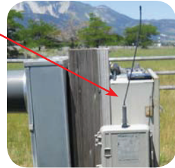
Photo of device with bent antenna.
