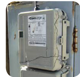
Photo of damaged device.
