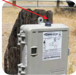
Photo of device with missing antenna.
