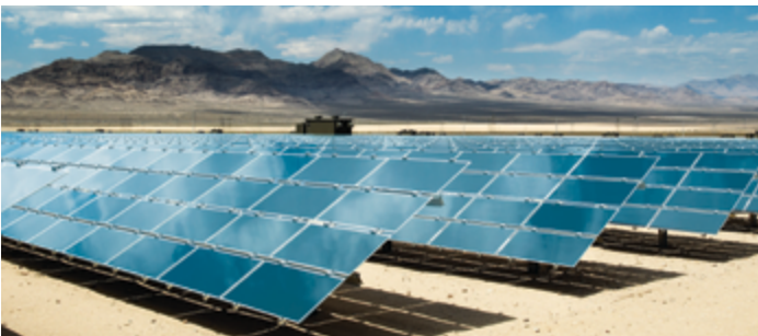
Silver State Solar North
