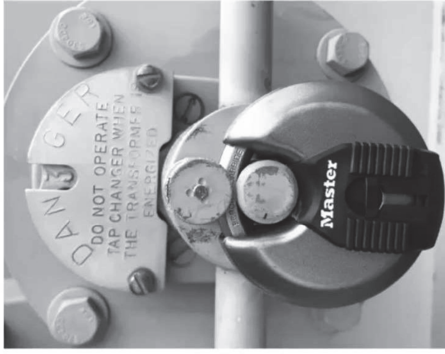
DETC with upgraded lock to hinder bolt cutters (E-ISAC)
