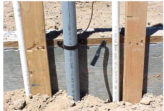
Figure 4 Conduit Support Strap Attached To Sill Plate
