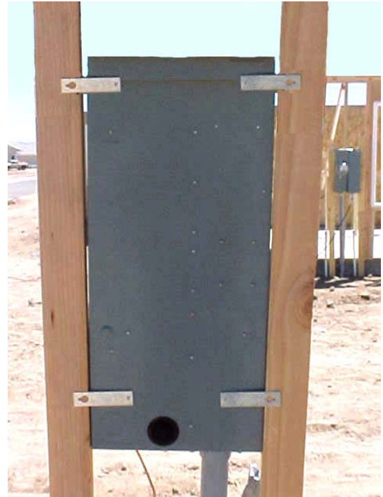
Figure 3 Panel Back Showing Swing Out Mounting Brackets Attached To 2"x4" Stud Framing
