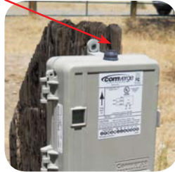
Photo of device with missing antenna.
