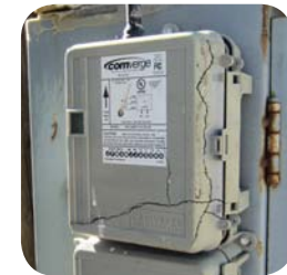
Photo of damaged device.
