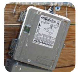
Photo of poor mounting.
