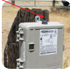
Photo of device with missing antenna.
