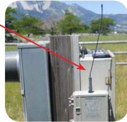
Photo of device with bent antenna.
