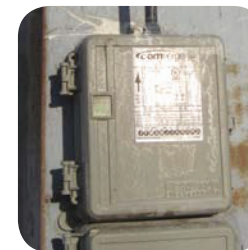
Photo of water damage.
