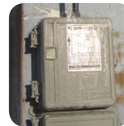
Photo of water damage.
