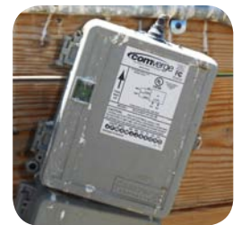
Photo of poor mounting.
