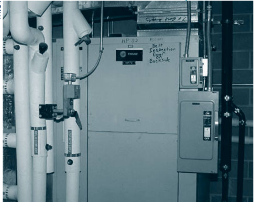
This commercial-sized GHP unit, installed in Cavett Elementary School, Lincoln, Nebraska, provides reliable year-round comfort.
