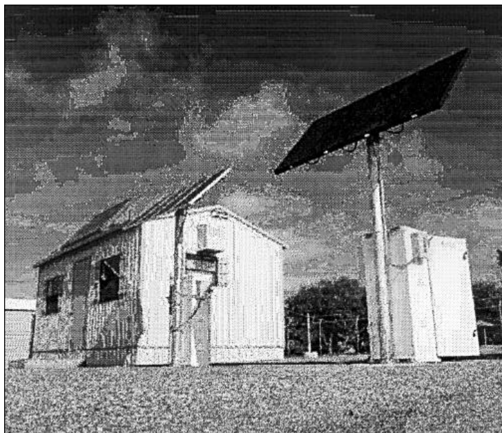
This stand-alone PV system consists of four modules, each with 36 cells. It provides power for lights, radios, televisions, and other loads at remote homes in New Mexico.
