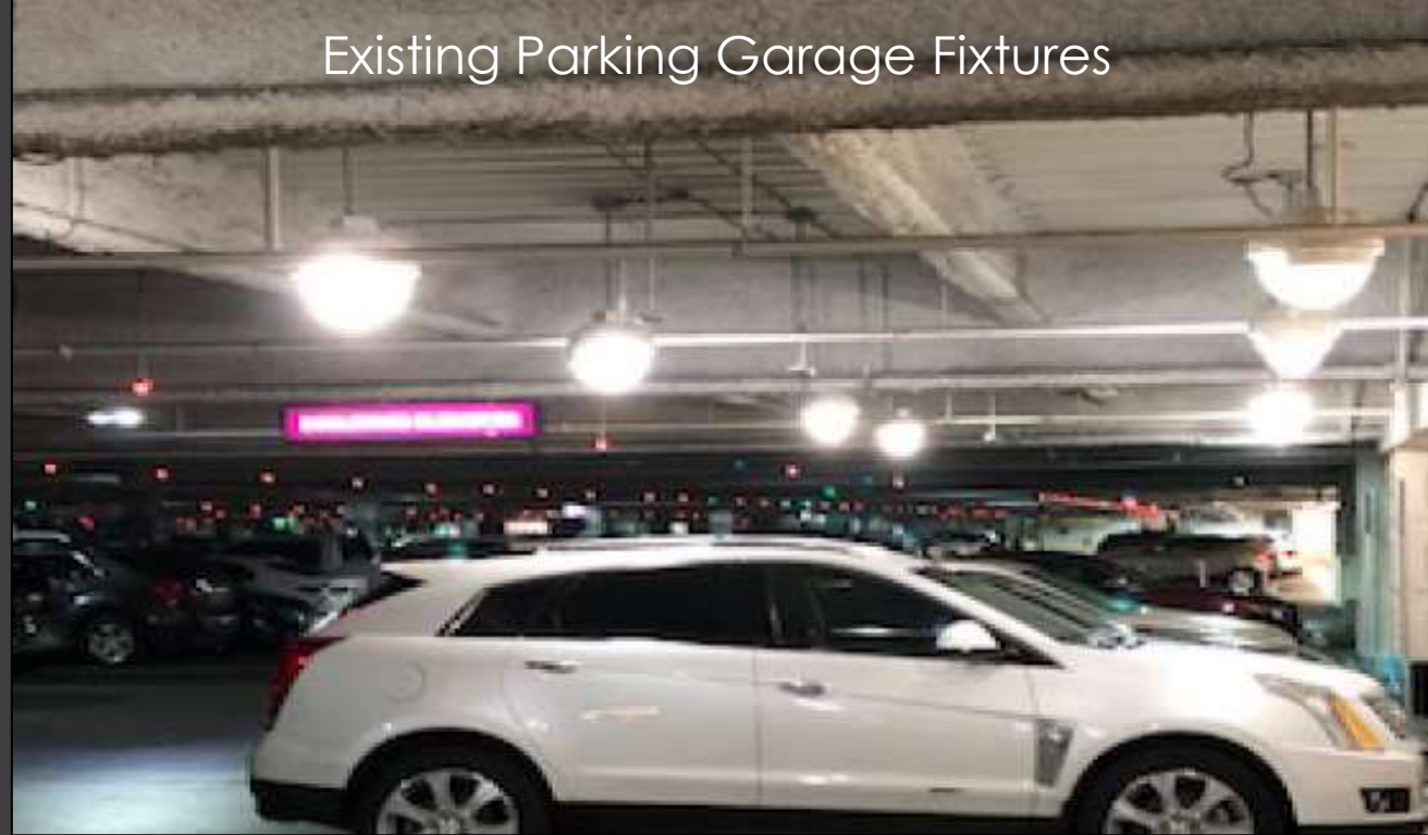
Existing Parking Garage Fixture Lamp
