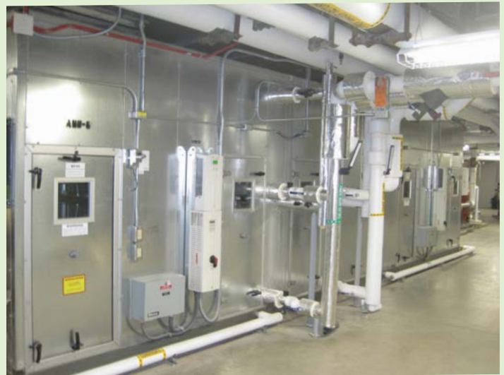
Large handling units benefit from variable speed drives
